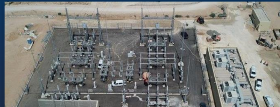
Oasis HV substation, Mashabei Sadeh
