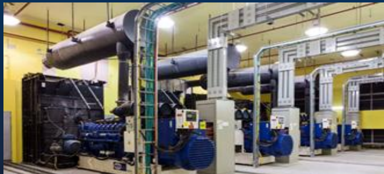
Med-1 Data Center, Petah Tikva
